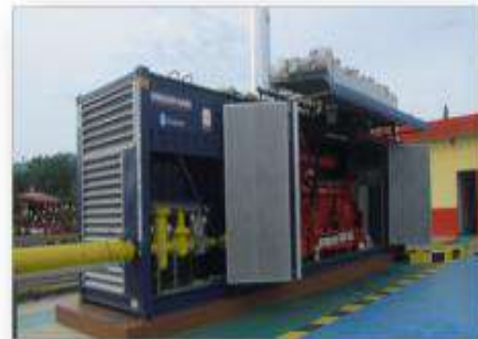
Umas Rural Electrification
