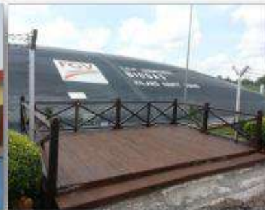
FiT Biogas Power Plant (15.4 MW) (11 units)
